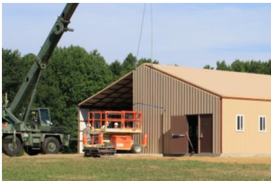
The final endwall is added. Trim and flashing are installed to complete the building.
