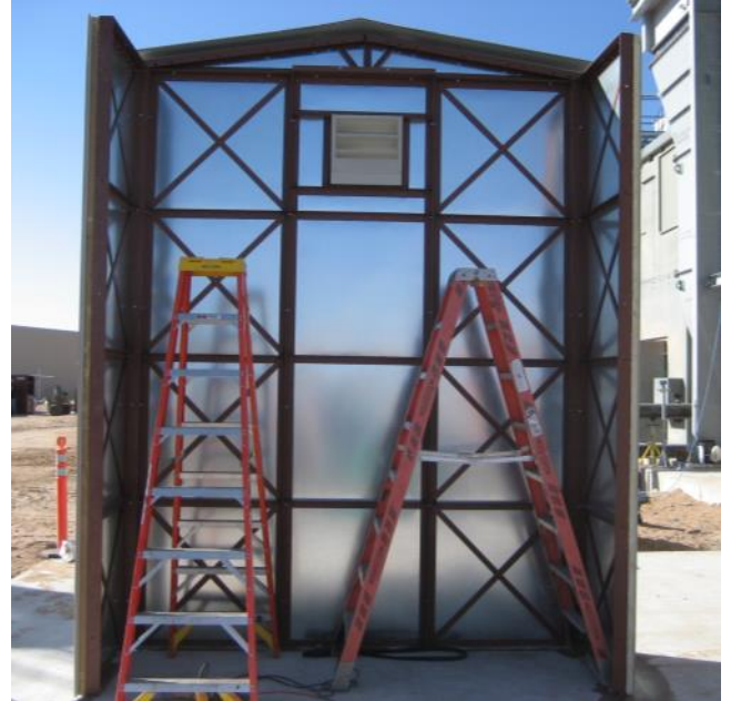
Additional panels create the first complete end-wall. A gable closure panel with factory attached trim creates the start of the gable roof shape.
