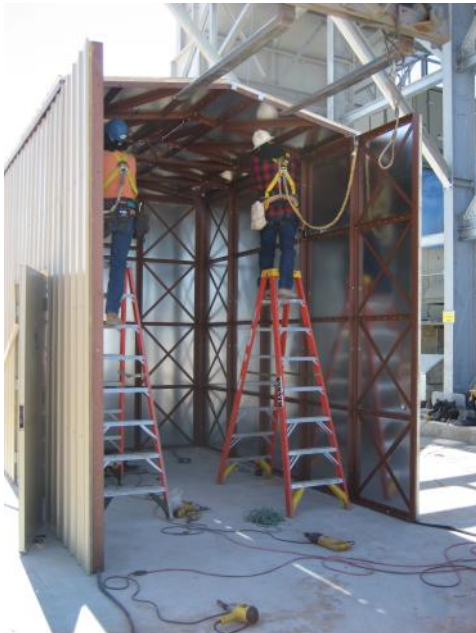
Roof panels are hinged at the ridge. The roof structure is completed with roof trusses comprised of a tension tie and web braces that bolt to the roof panel in the air.
