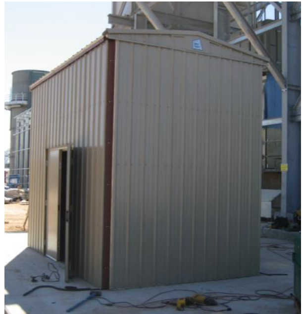
The final endwall installs similar to the first end-wall. Standard trim and flashing is installed to complete the exterior.
