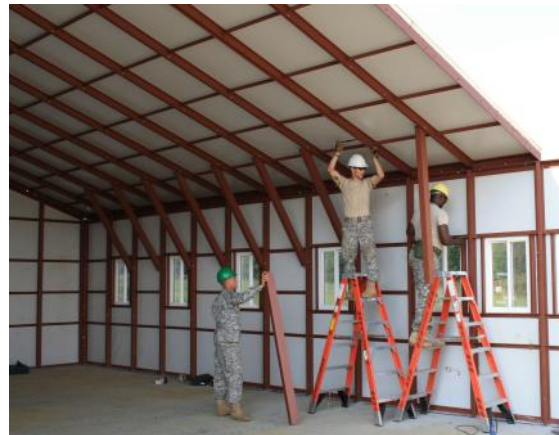
Knee and ridge braces are installed as wall and roof panel sections are set in place.
