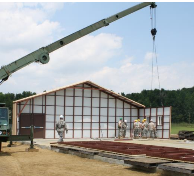
Sections of sidewall panels are sub-assembled and lifted into place with the crane.
