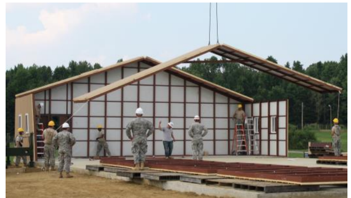
6' roof sections are assembled on the ground and lifted into place by the crane.
