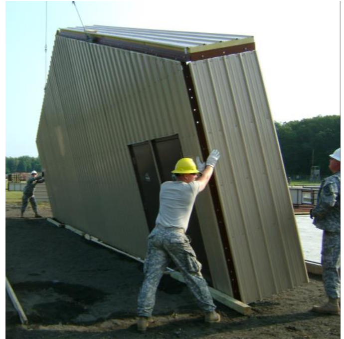
The endwall and 3' of sidewall and roof are lifted into place with a crane.
