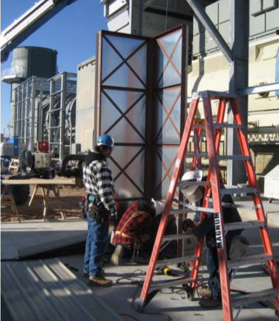
Two wall panels and a corner erection angle make the first corner of the building.
