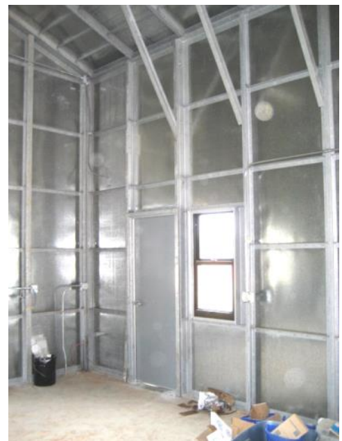
A Building's Interior with Hot-Dip Galvanized Frames in the Gulf Coast Region
