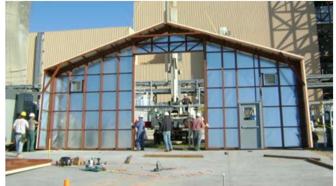
Endwall Being Set with Factory Installed Personnel Door, Louvers and Equipment Door Supports
