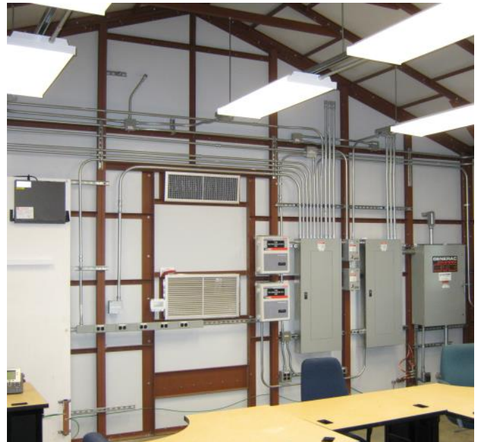
Interior View of Factory Installed Wall-Mount HVAC Framing
